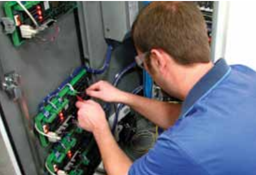
Service technician, Orion Smith, checking voltage of a MPLC card (Motion Programmable Logic Control).
